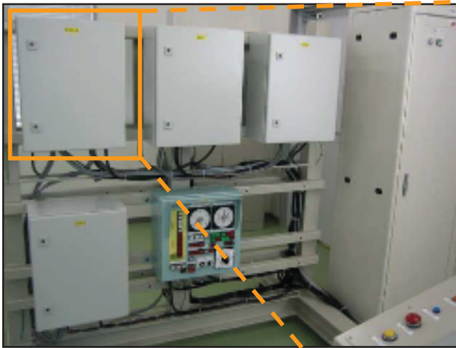
Cabinet for MPC
