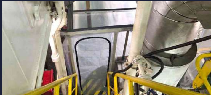
Enclosure of engine room
