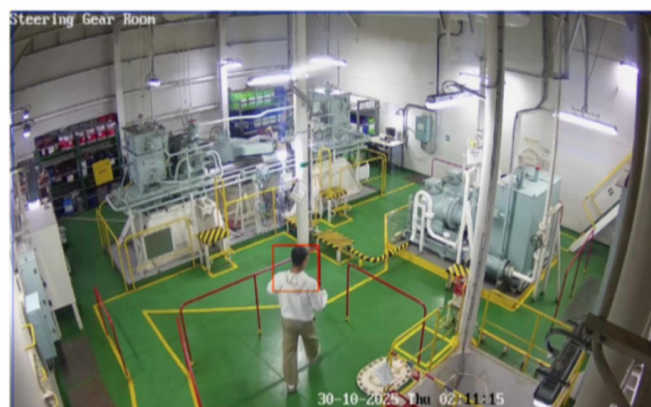
Channel: Steering Gear Room
