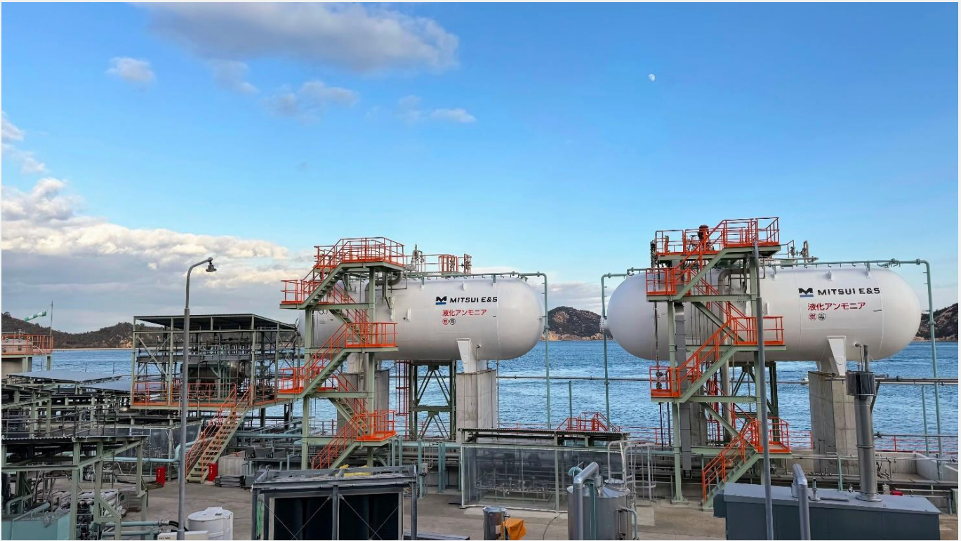
Photo 2: Ammonia Fuel Supply System (onshore)
