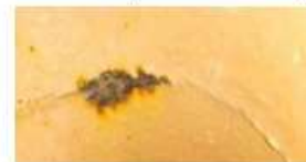
Picture 3 Paint peeled off at butt-welded parts of distance pieces
