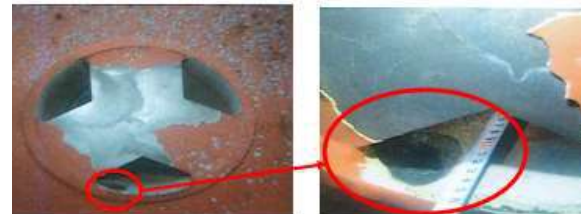
Picture 2 Corrosion on/around welded parts between distance pieces and bluff bodies
